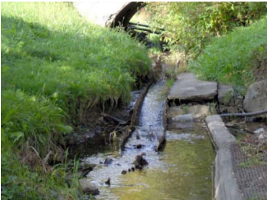
Figure 3. A) Perched culverts. B) Debris restricting the stream. These are examples of fish barriers found in the Niagara River Area of Concern (AOC) - Fish Barrier Project (Niagara Restoration Council, Niagara Peninsula Conservation Authority, 2007)
