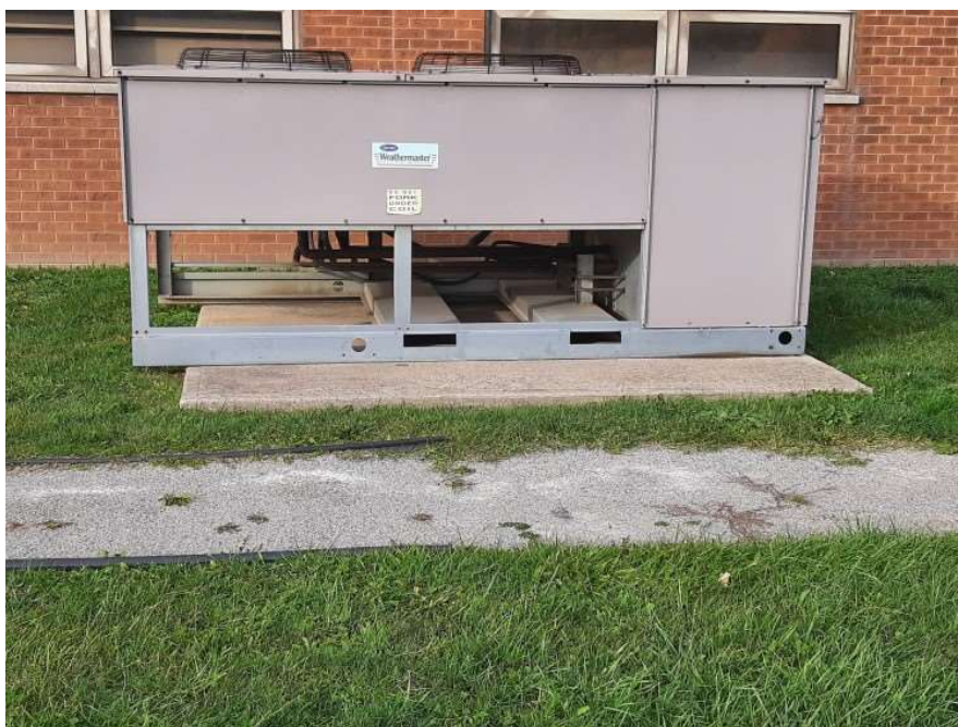
An HVAC system.
