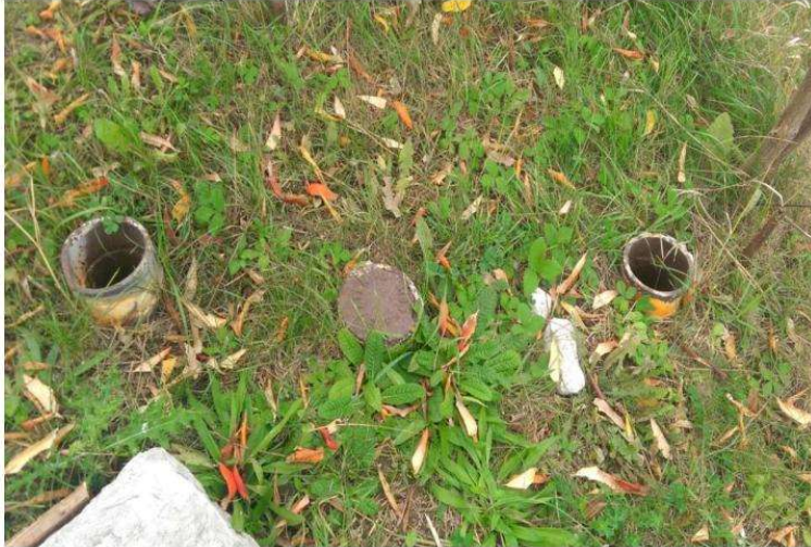
Appendix B – Photo 11. Unknown pipes on Northwest side of the North Lagoon, near the First Nations Garden.
